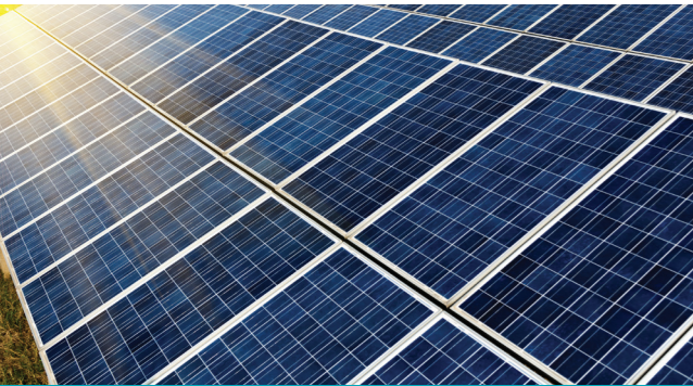
PICTURE 3 | Solar energy plant
