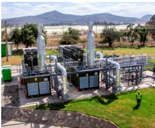
Biogas plant in Kenya. (Source: VP Group)
