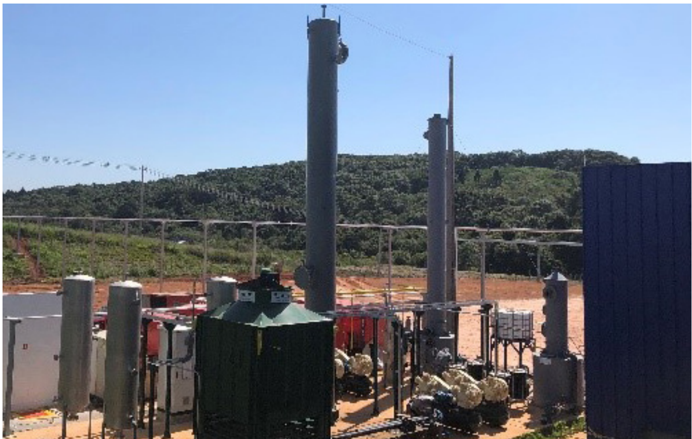
Biogas treatment plant in Brazil. (Source: Castrolanda)
