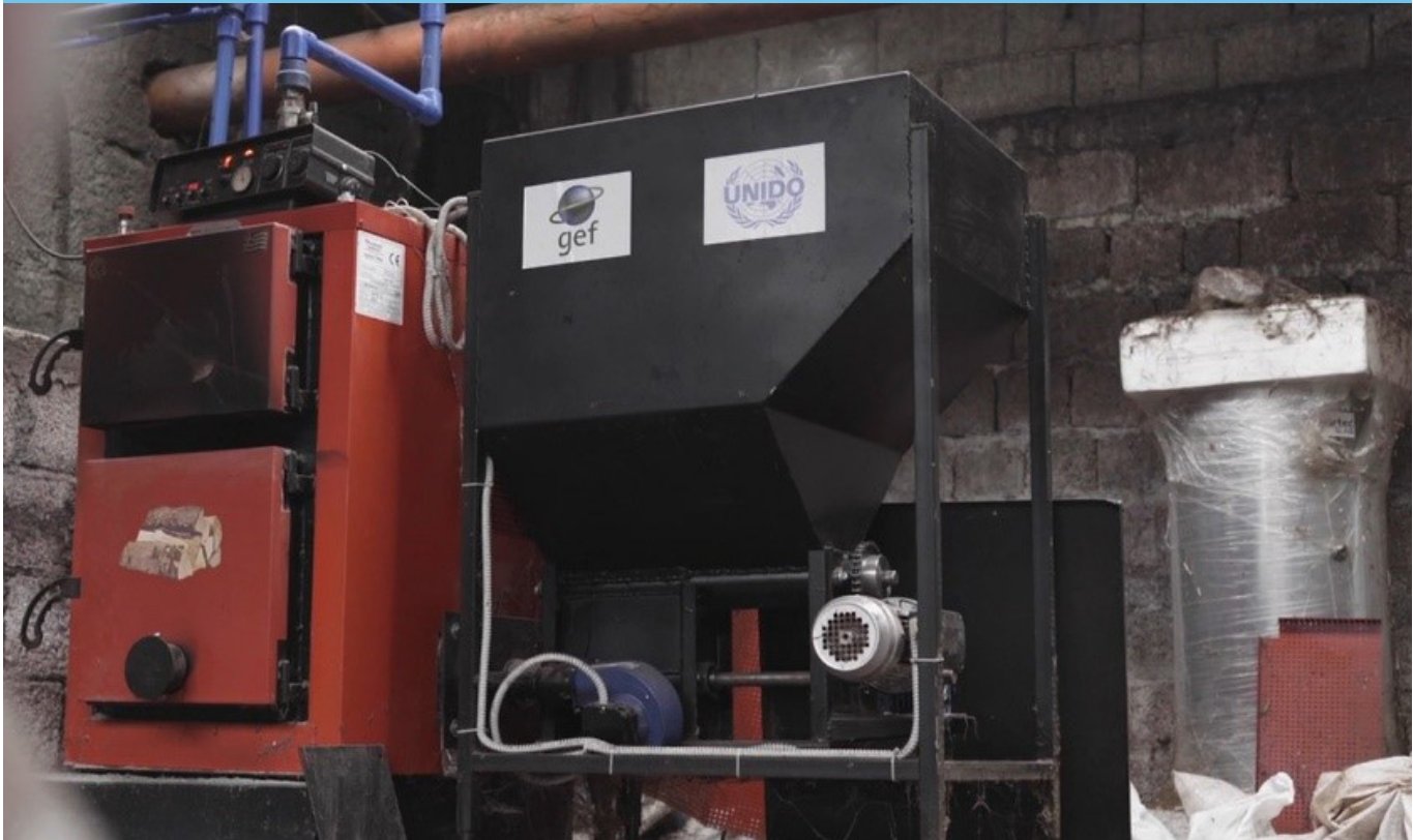
Combustion system for dried olive pomace in an olive factory. (Source: BEA)
