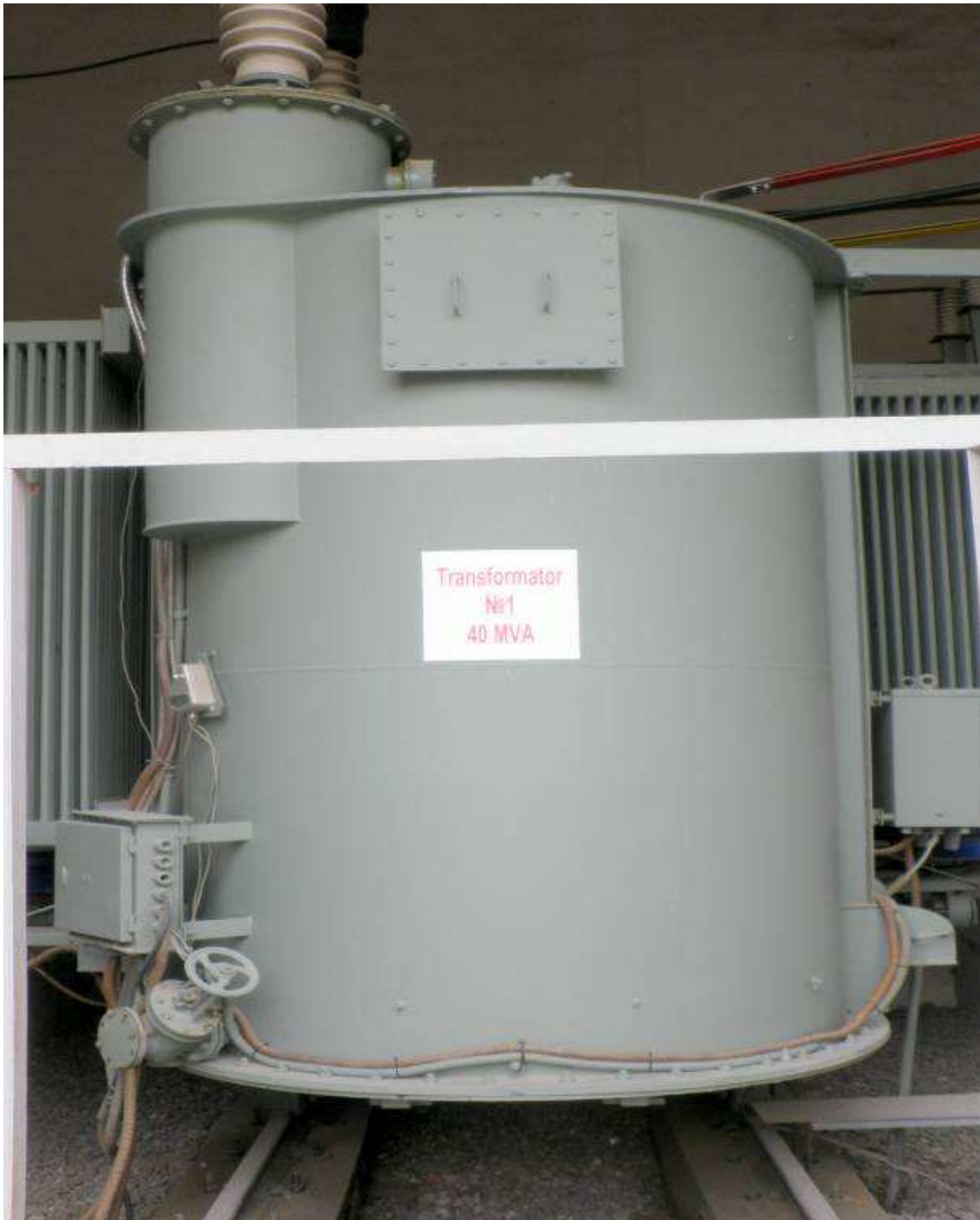
Picture 15. One of the transformers at Bakuelektrik.
