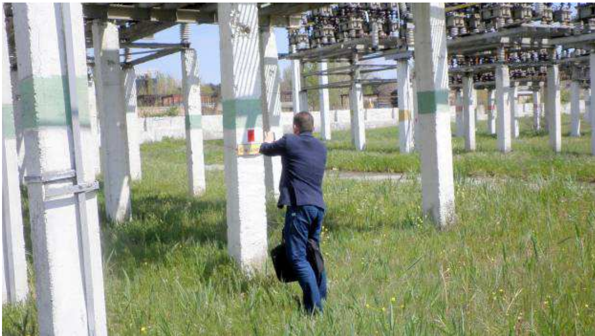
Picture 4. The labelling of the capacitors. When the label is red it means that after the analysis is discovered that the capacitor contains PCB oil. The label is green when it is ascertained after the analysis that the capacitor is free of PCB.
