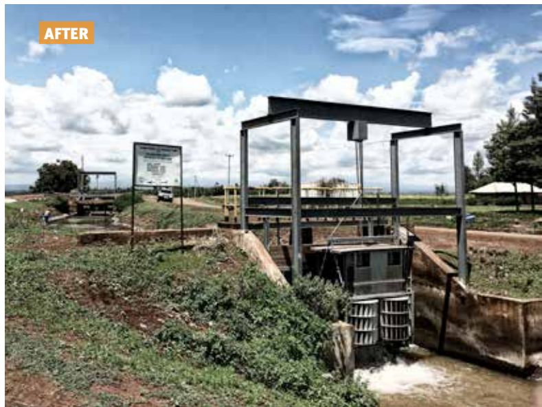
BEFORE AND AFTER INSTALLATION OF THE ULH-MHP AT THE MWEA IRRIGATION SCHEME CANAL
