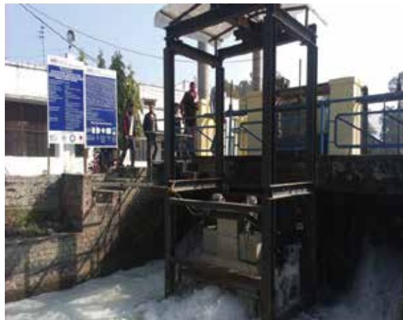
Figure 10: Ultra low-head micro hydro plant in Uttarakhand
