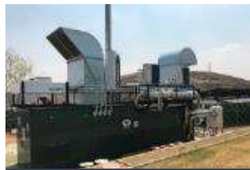
Power Generation with Methane Gas Recovery System, NTTDATA, Mexico
