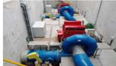
Hydro Power Plant, Toyo Energy Farm Co., Ltd., Indonesia
