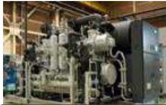
High-efficiency refrigerator, Mayekawa MFG, Indonesia
