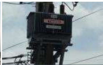
Amorphous transformers in power distribution, Hitachi Materials, Vietnam
