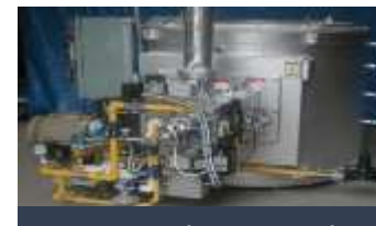
Regenerative Burners in industries, Toyotsu Machinery, Indonesia
