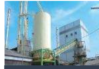
Biomass Co-Generation System, Fuji-Foods Coporation, Thailand
